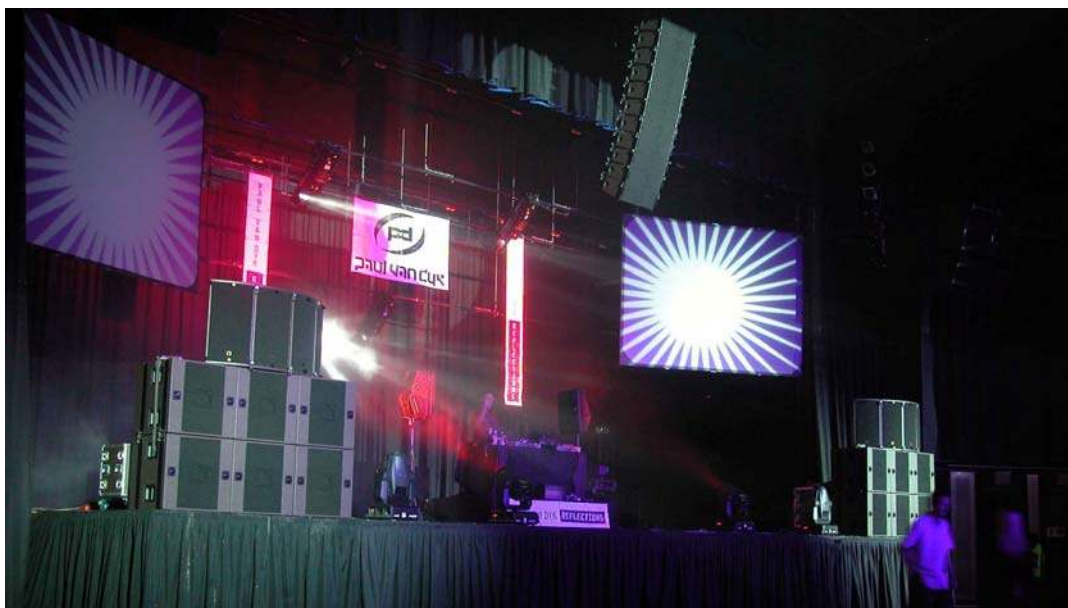
Figure 25: Stacked ARCS FOH system (including dV-SUB and dV-DOSC centre cluster)
